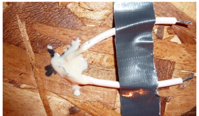
Figure 4 Resistance Temperature Detector Secured with Thermal Urethane in the Attic
