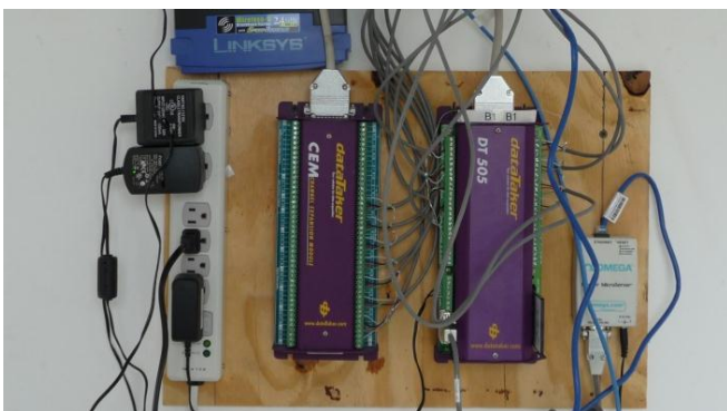
Figure 6 Data Logger Installed Inside of Control (500 Unit)
