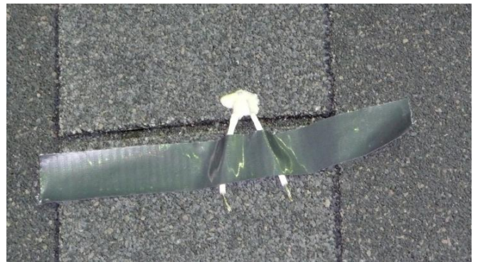
Figure 3 Resistance Temperature Detector Secured with Thermal Urethane on the Roof
